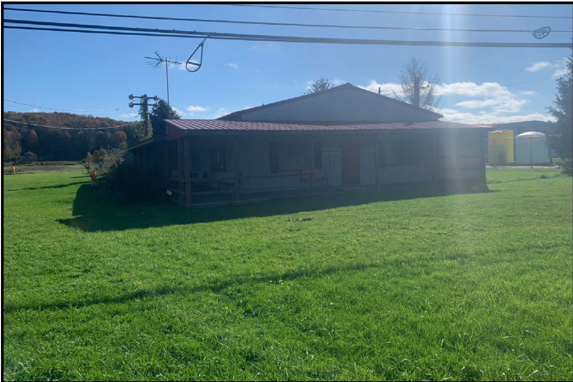
Photo 4. Facing southeast along NYS Route 16/98 showing field conditions, field methodology, and the commercial building to be demolished.
